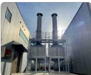
Odor treatment facility (A***, Osan plant)
